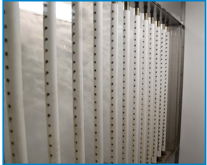
Condensate from the Ultra-sorb XV dispersion panel is never wasted; it is flashed back to humidification steam by a heat exchanger in the header.
