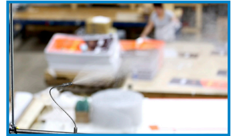
One of the 165 atomizing nozzles in over a quarter mile of tubing throughout Modernistic's 160,000-square-foot facility.
