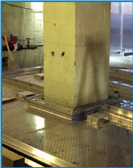
Structural column incorporated into air handler design
