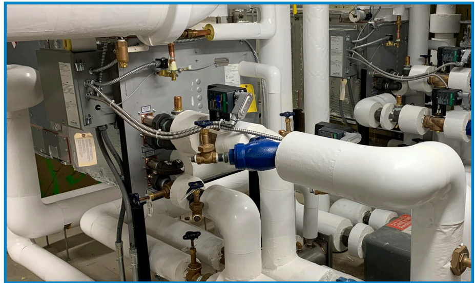
Two DriSteem STS steam-to-steam humidifiers, each capable of 1 600 pounds per hour of clean humidification steam
