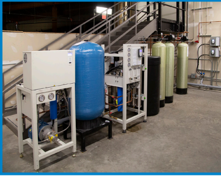
Mechanical room where water is purified and pressurized before it is pumped to the dispersion nozzles near the Rogers Place ceiling
