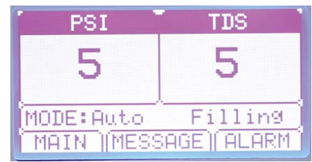
FIGURE 16-1: RO STATION KEYPAD/ DISPLAY HOME SCREEN
