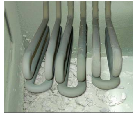
FIGURE 20-1: HARD WATER SCALE ON HEATERS AND TANK
