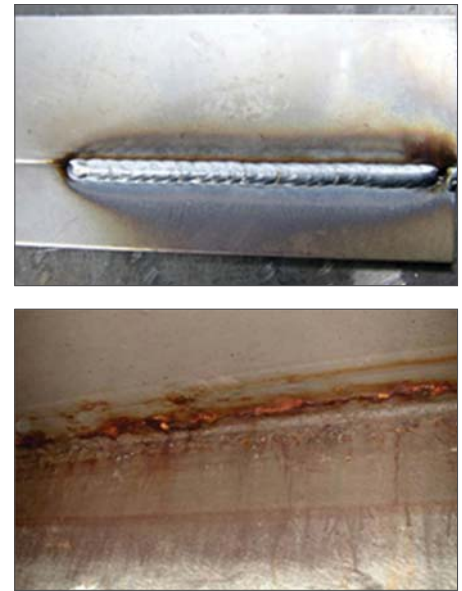
FIGURE 42-1: STAINLESS STEEL CORROSION EXAMPLES
