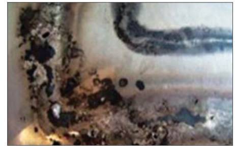
FIGURE 46-1: CREVICE AND PITTING CORROSION
