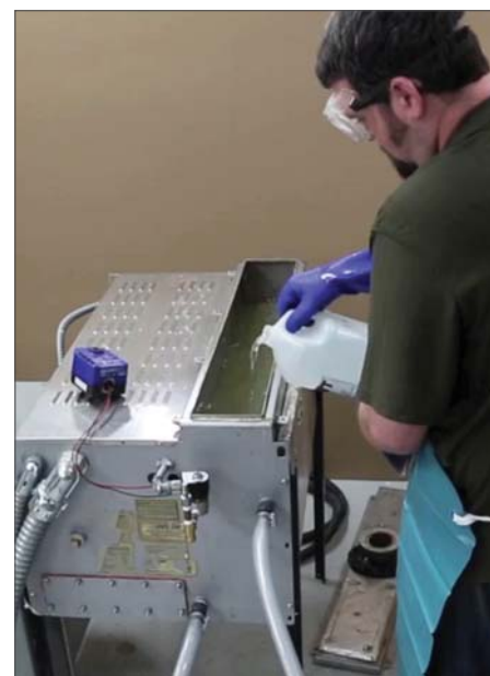
FIGURE 9-2: POURING DE-SCALING SOLUTION INTO A HUMIDIFIER TANK
